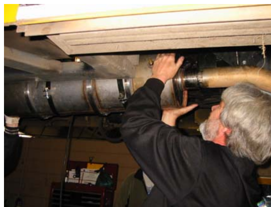
Mechanic Installing a DPF on a Bus by Simply Replacing an Existing Muffler
